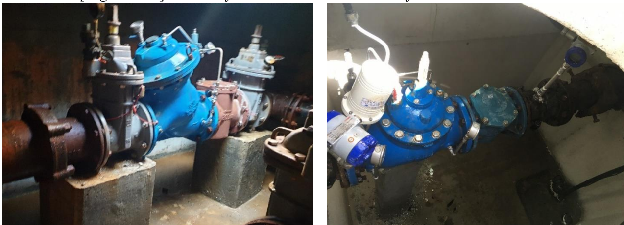
[Figure 2-12] A View of Local Water Pressure Relief Valve in Seosan-si >
