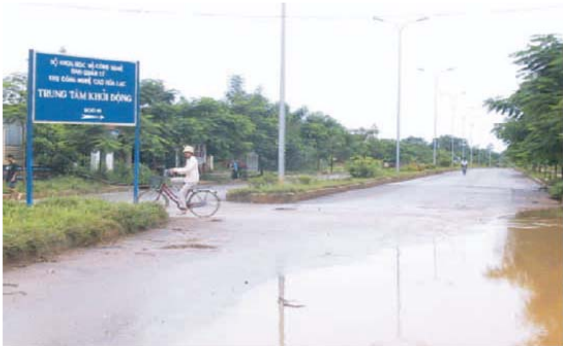
Figure 30 Insufficient infrastructure in HHTP
